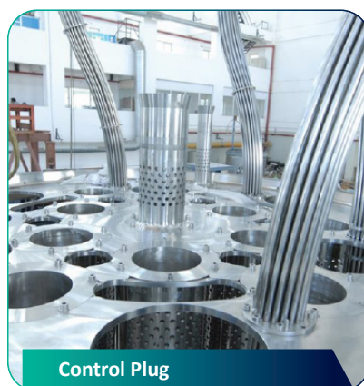
Calandria Vault Top Hatch Cover Beam
