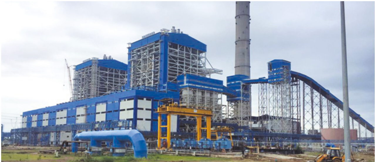
NTPC 800MW Super Thermal Plant, Gadarwara
