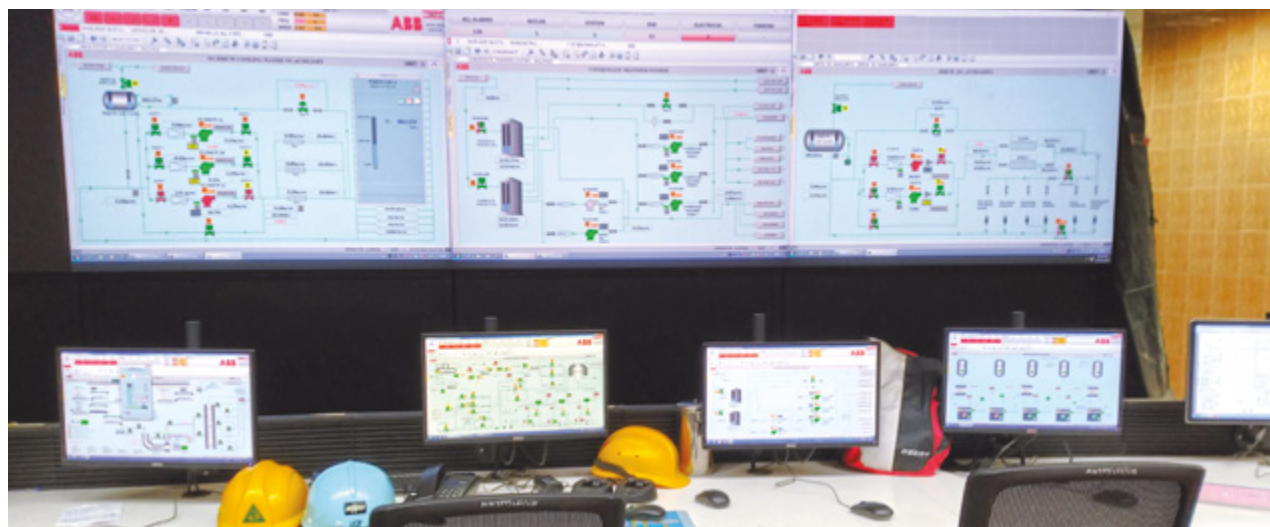
Neyveli 2x500MW - Control Room
