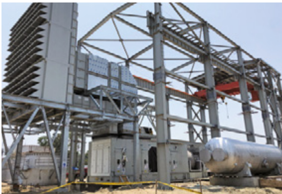
Shajibazar – Power Block
