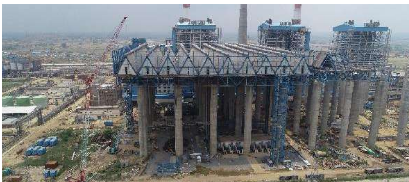
Air cooled condenser, NTPC North Karanpura
