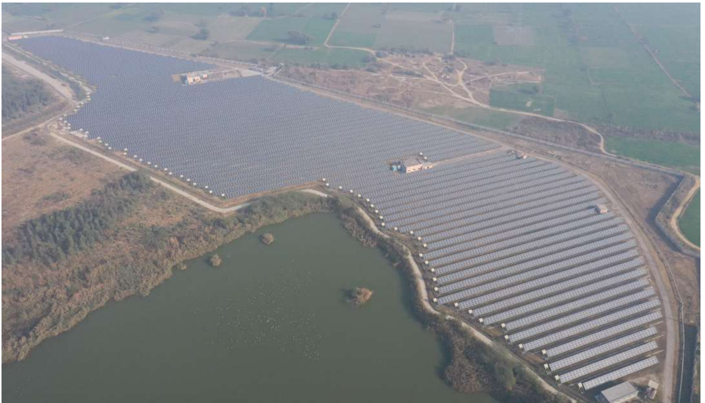
NTPC Solar Andaman
