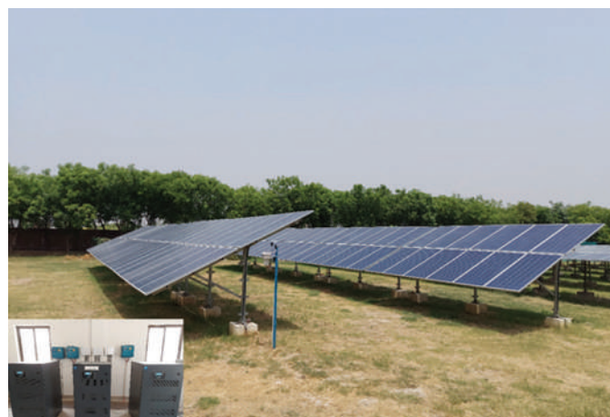
30 KWP DC Microgrid, NETRA
