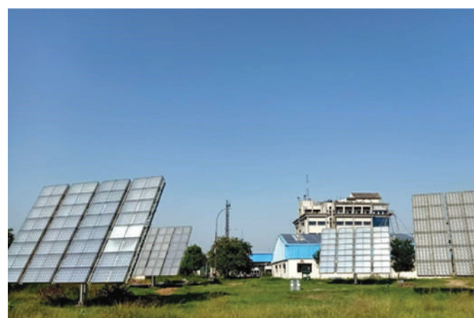
53 Kw Concentrated Photovoltaics Module setup, NETRA
