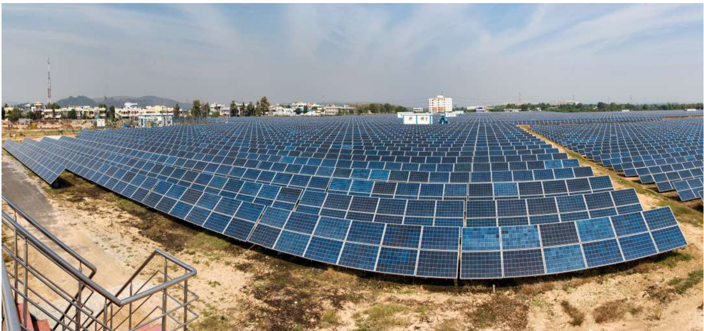
NTPC Solar at Ramagundam
