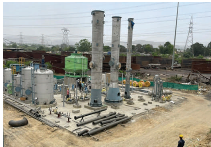
20 TPD Carbon Capture Plant, Vindhyachal
