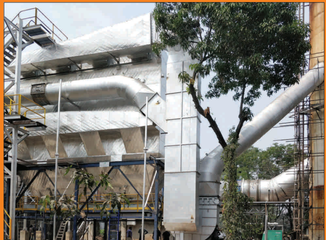
State-of-the-art Dust Extraction System.
