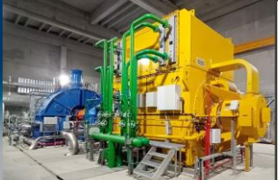
Steam Turbine Generator & Site Installation
