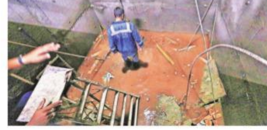
Elevator of the building collapsed Wednesday. Nirmal Harindran
