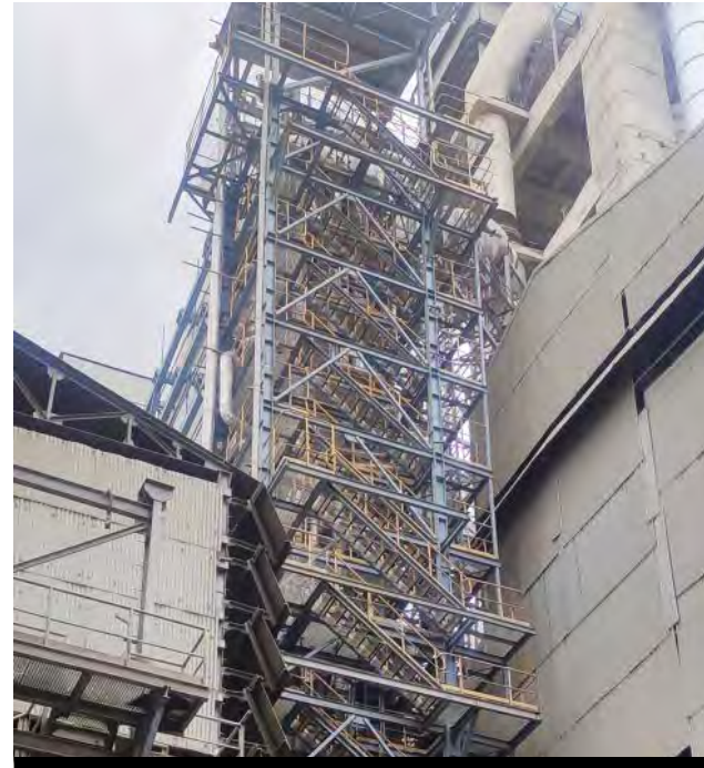
P H Boiler
