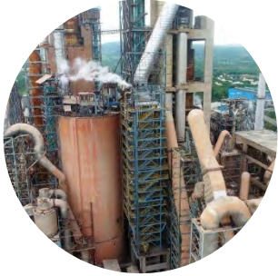
Waste recovery system (WHRS)
