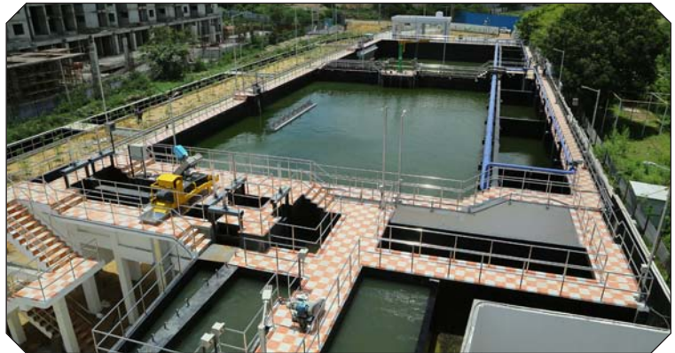
Sewerage Treatment Plant, Kokapet, Hyderabad, Telangana
