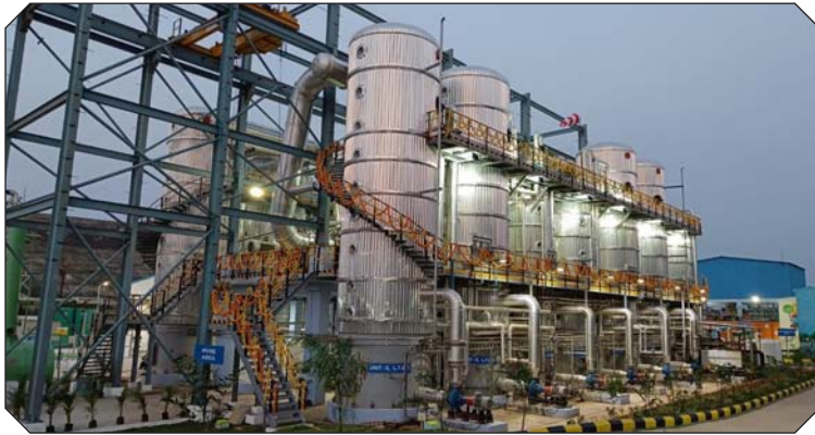
Jawahar Nagar Leachate Treatment Plant Hyderabad, Telangana
