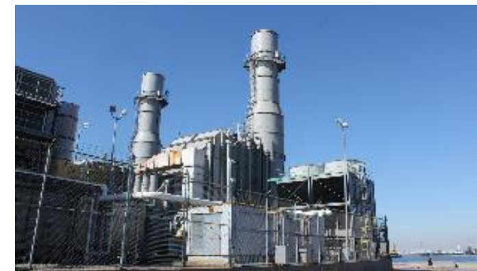
Captive Thermal + Waste Heat Plants (Total capacity of 161.5 MW)
