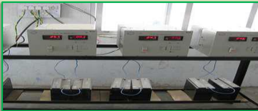
Battery and Battery Chargers
