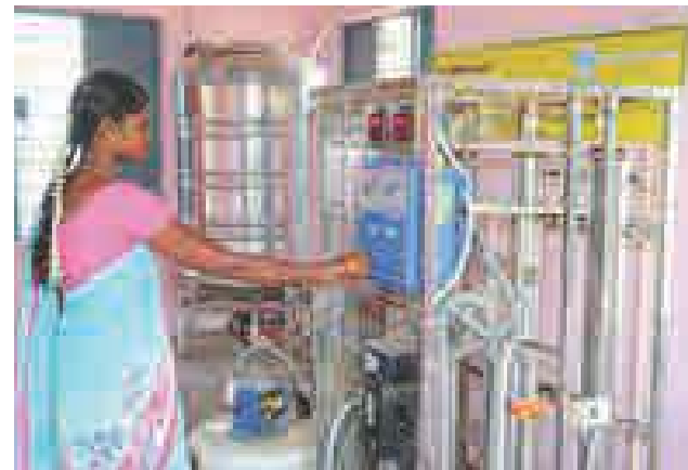
Community RO plant at Malaipattu village, Kancheepuram
