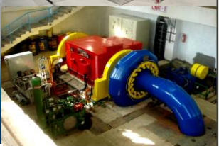
Hydro Turbine Generator & Site Installation
