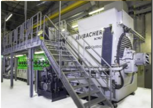
Gas Engine Generator & Site Installation
