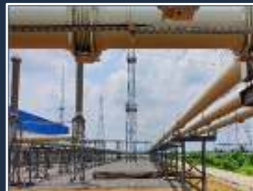
Eighteen bays of 400 kV GIS with 3600 meters Gas Insulated Busbar for L&T at Thallayapalem in Andhra Pradesh
