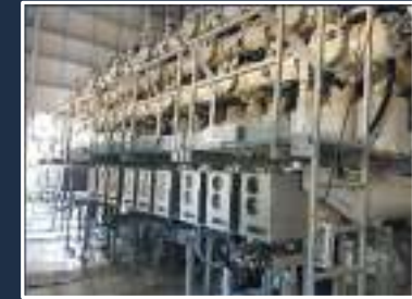
220 kV bay along with 220/34.5 KV, 50 MVA Transformer commissioned at NTPC Uncharar
