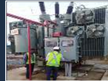
21.6 MVA, 132/27kV TSS Transformer commissioned for National Mineral Development Corporation at Nagarnar
