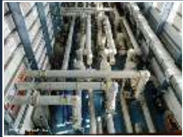
Four bays of 765 kV Gas Insulated Substation (GIS) with six 765 kV Line Reactors commissioned at Vadodara for LVTL Sterlite Power Transmission limited
