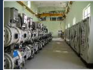
132 kV GIS at Ramnagar for West Bengal State Electricity Transmission Company Limited
