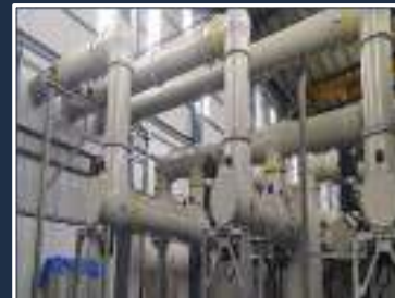
Six bays of 220 kV GIS with 1200 meters Gas Insulated Busbar for Sterlite's project for PGCIL at Vadodara Gujarat
