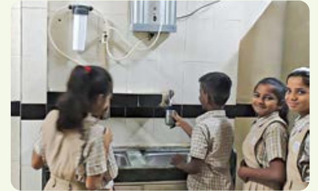
Water Dispenser Installed in School under CSR
