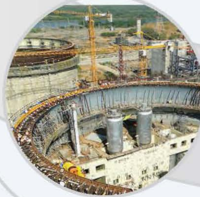
Main Plant Electrical Package for 2 x 700 MWe Kakrapar Nuclear Power Project
