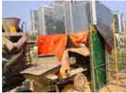
Use of rockwool insulation- Noise Pollution mitigation (Mahindra Luminare, Gurugram)
