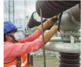
Switchyard Maintenance at Dhule Substation
