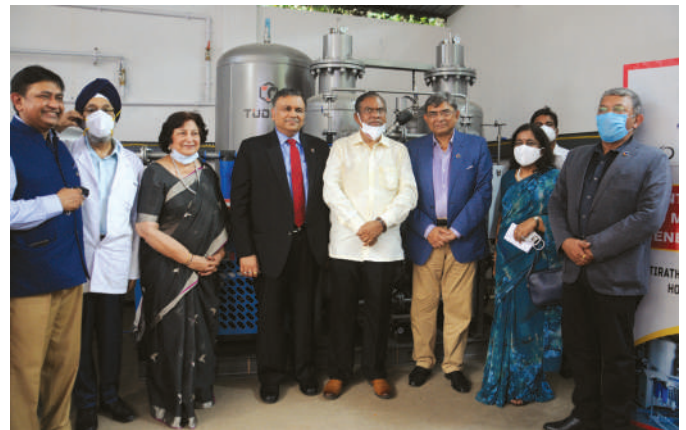
Oxygen plant set up at TRSCH, New Delhi to strengthen healthcare infrastructure and partner the fight against COVID-19
