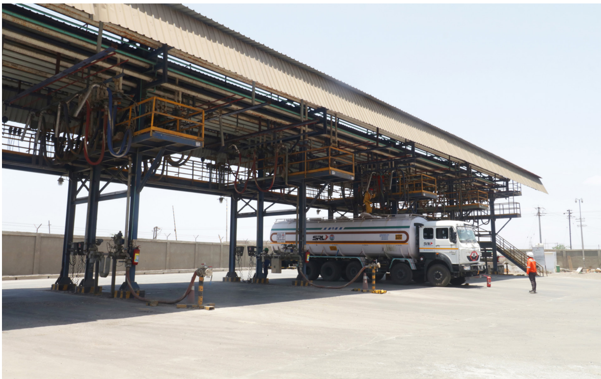
Tanker loading in Progress
