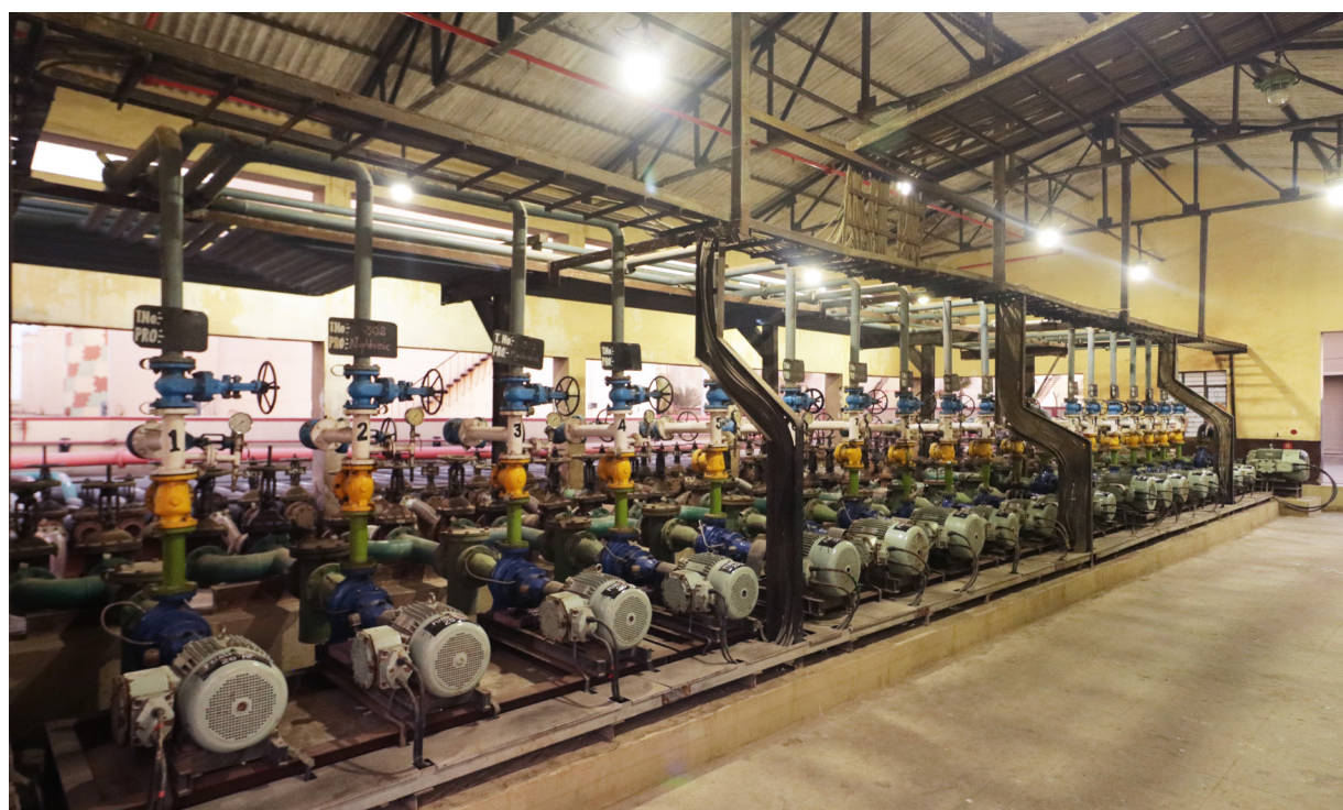
Pump house at Kandla terminal
