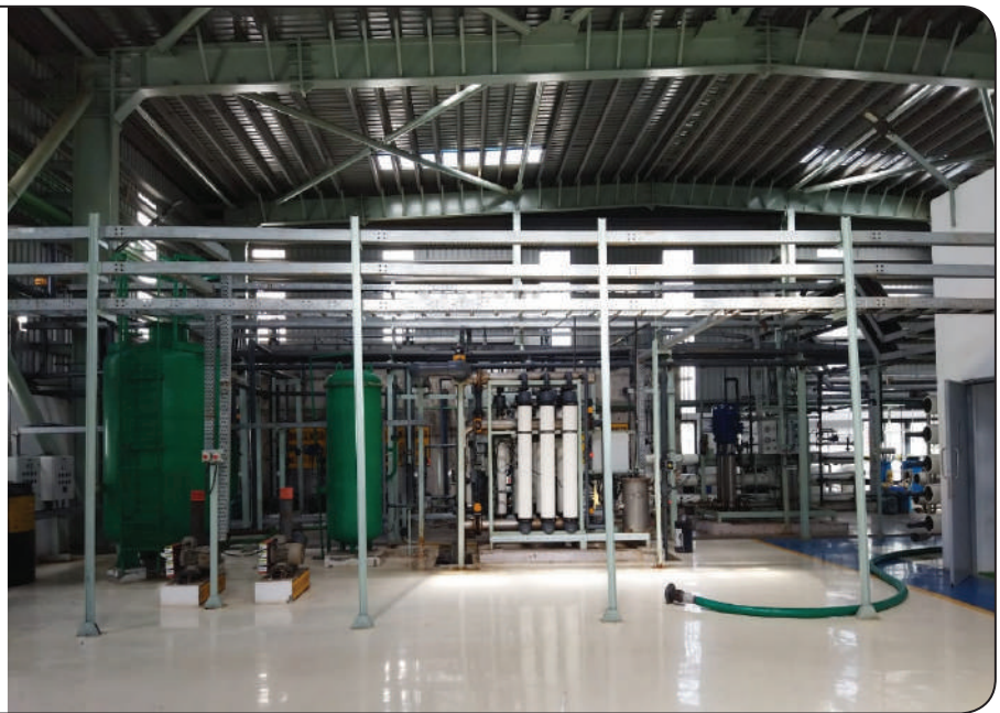
Effluent Treatment Plant
