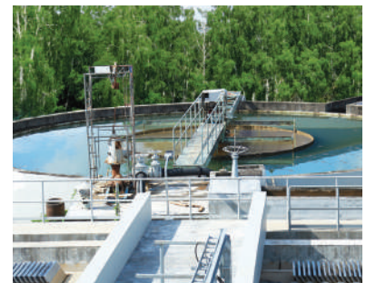
Clarifier Capacity: 660 m 3 /h
