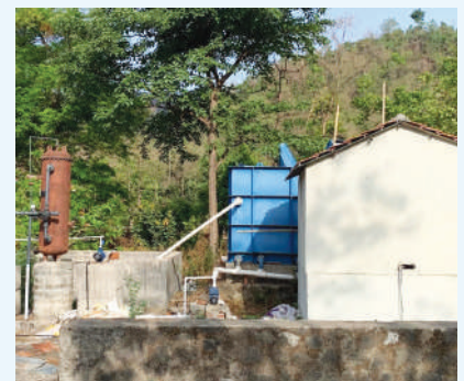
Setting up of Water Treatment Plant (WTP) & Sewage Treatment Plant (STP), Om Creations Trust, Maharashtra
