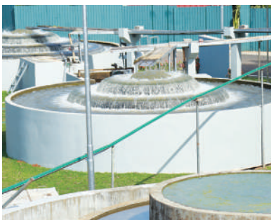
Cascade Aerator for UHRSCC Flow rate: 800 m 3 /h
