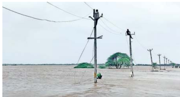
Power line being repaired at Ghed village in Junagadh on Tuesday, following heavy rain. Express
