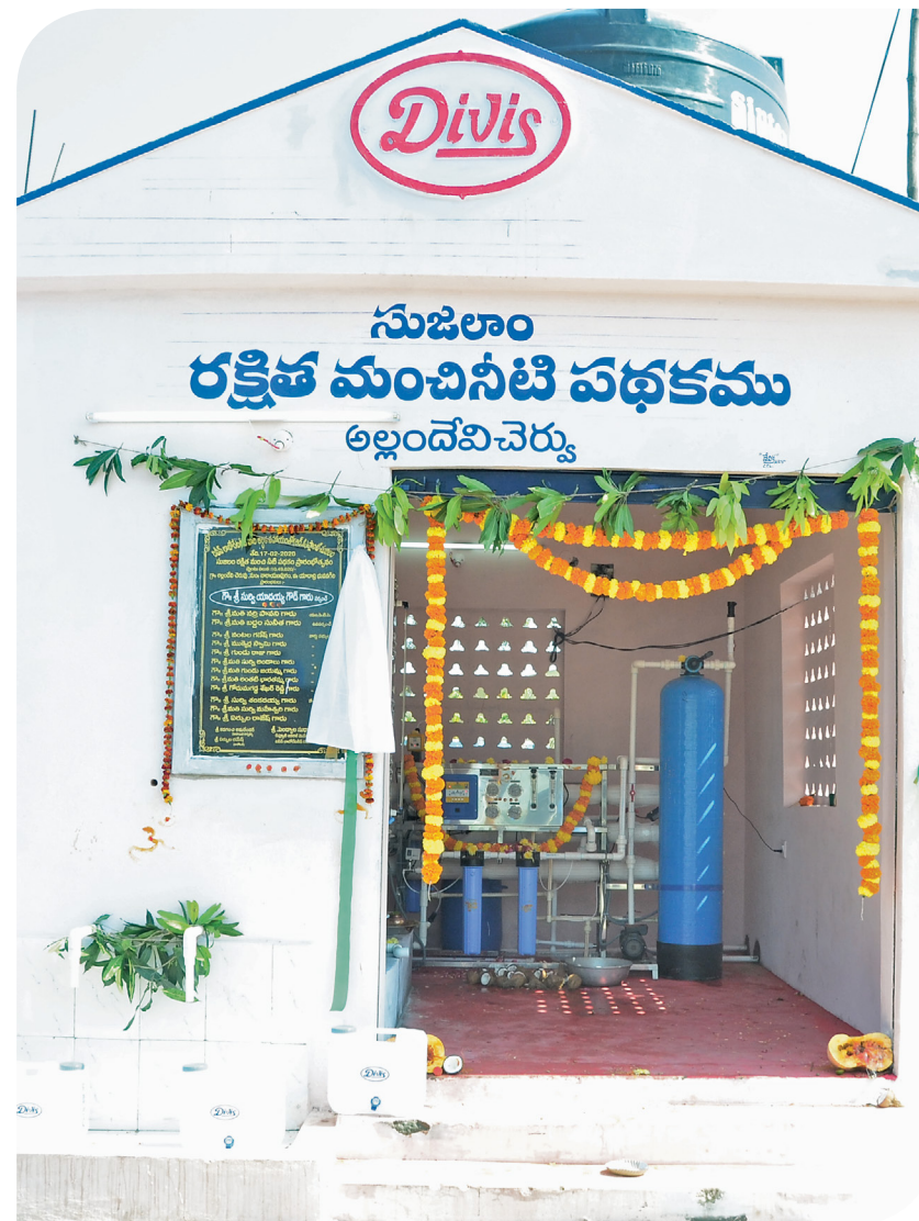
RO plant installed at Allamdevi Cheruvu - Visakhapatnam
