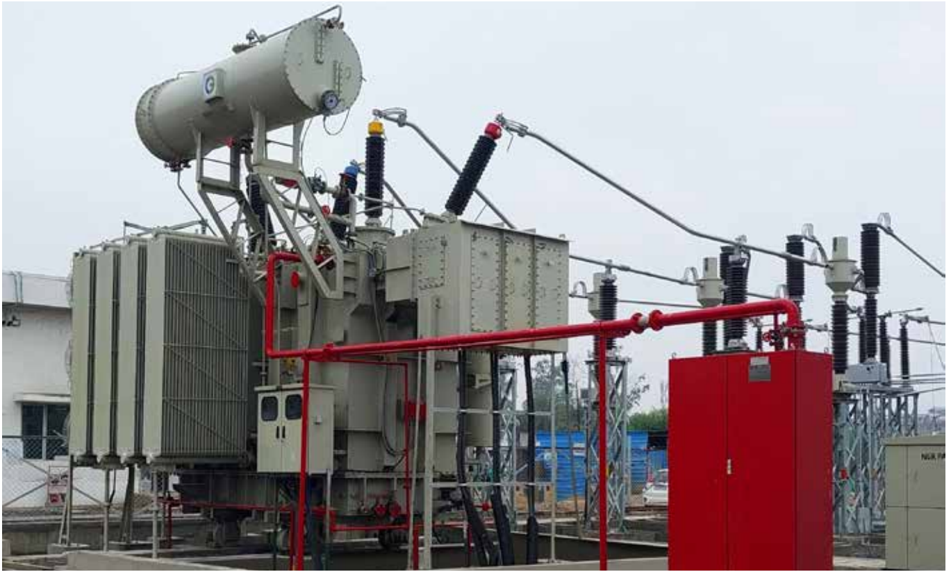
50MVA 132kV Power Transformer Supplied by CG for Bhopal Metro Project
