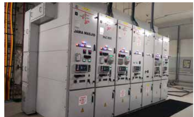
33kV GIS Supplied by CG for Underground Substation, UPMRCL, Agra Metro Project
