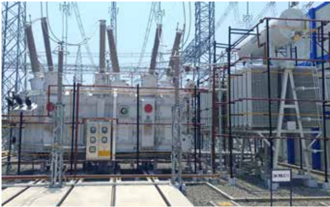
500MVA 400kV 3-Ph ICT Supplied by CG for Karur Substation Project
