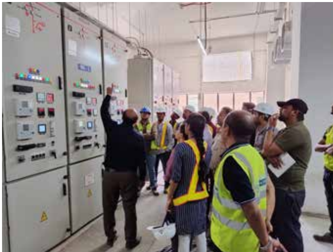
33kV GIS Supplied by CG for Mumbai Metro - Aarey Depot Project
