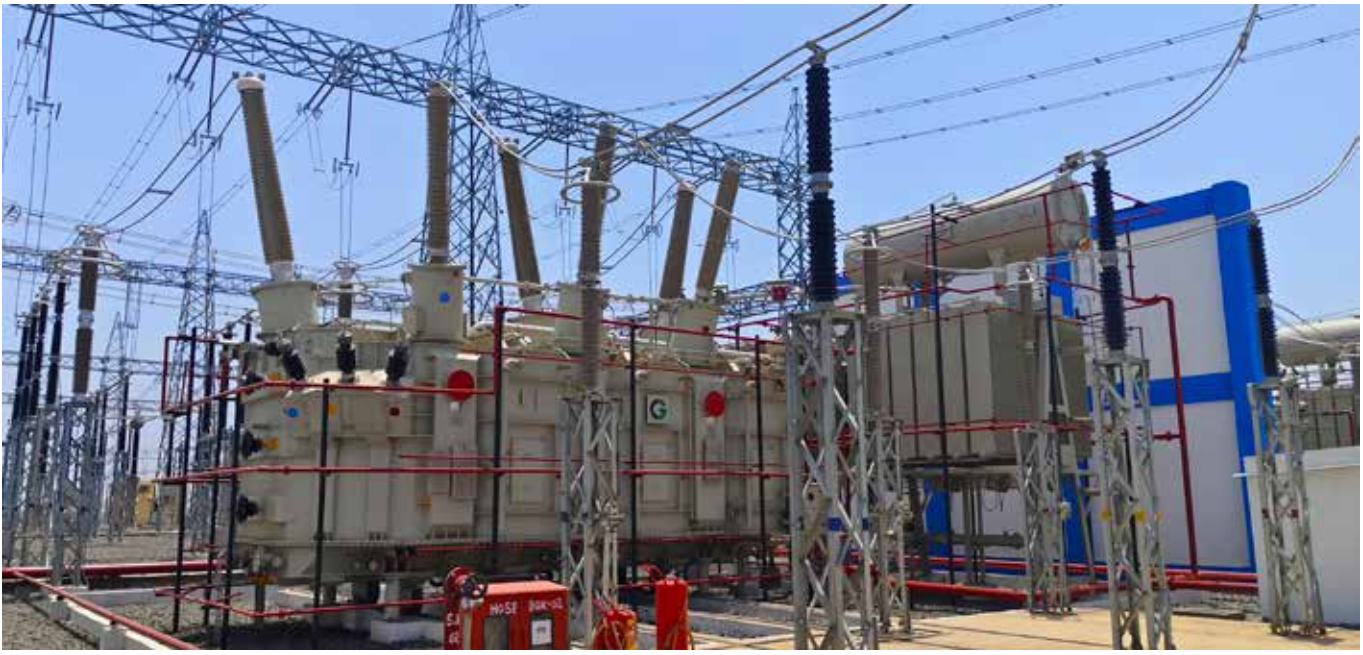
500MVA 400KV 3-Ph ICT Supplied by CG for Agar Malwa Substation Project
