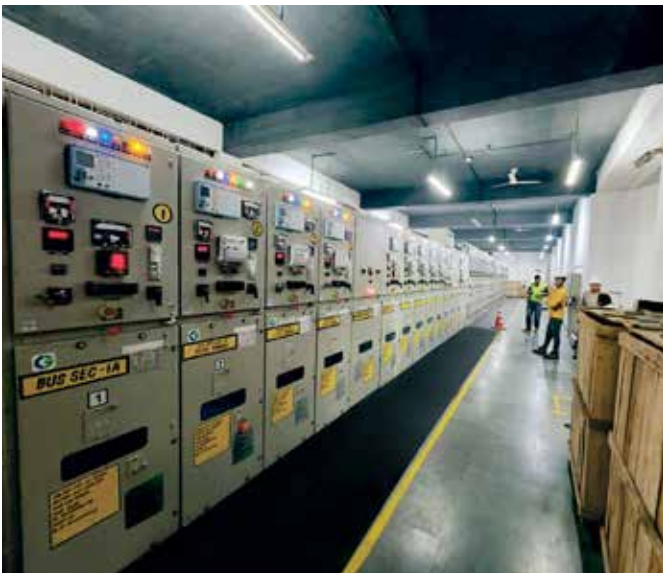
11kV VCB Panels Supplied by CG at Tata Power Delhi Distribution Ltd. (TPDDL) Unmanned Substation, Bawan Grid
