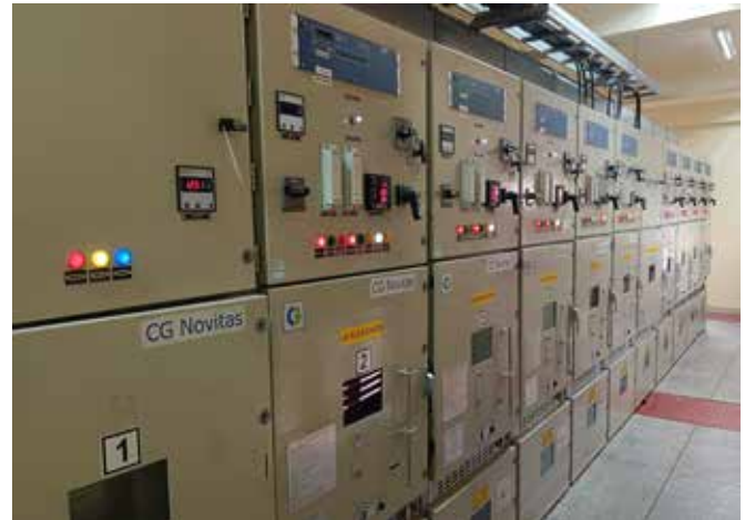
12kV VCB Panels Supplied by CG at Gandhi Village Substation Trinidad and Tobago, West Indies
