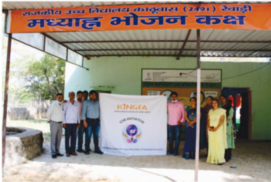
Construction of Tin Shed for Mid-day meal at Govt. High School, Kathuwas, Rewari- ₹ 1.89 Lakhs
