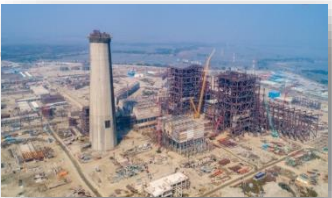
2X660 MW at Rampal, Maitree, Bangladesh-BIFPCL
