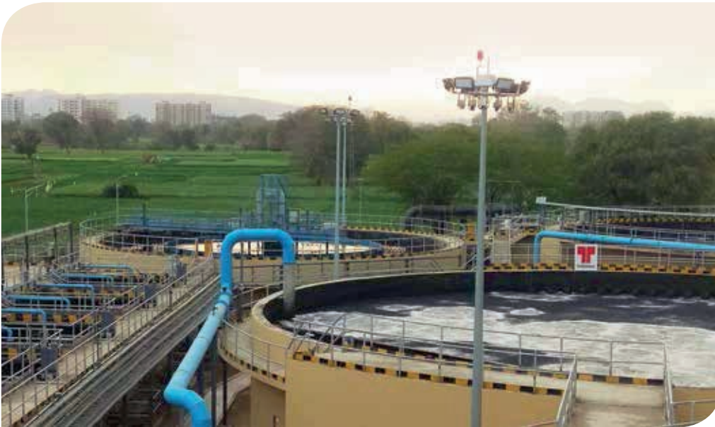
The Water & Waste Solutions business of Thermax commissioned a Sewage Treatment Plant of 25 MLD (million litres per day) capacity at Udaipur for the world's leading zinc-lead-silver producer.
