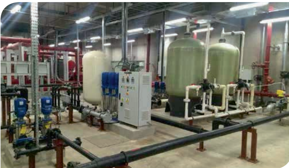
A Water Treatment Plant commissioned by Thermax for a Swedish furnishing major's first store in India. The plant produces 2,000 litres of treated water per hour, catering to the potable and non-potable water requirement of the entire store.
