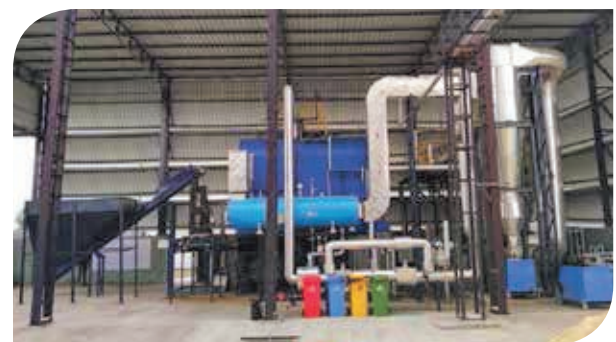
Combloc UFS 30, a 3 TPH boiler installed in Maharashtra for a German multinational producing animal feed. This biomass fuel-based boiler is semi-automatic, designed for small-sized plants.
