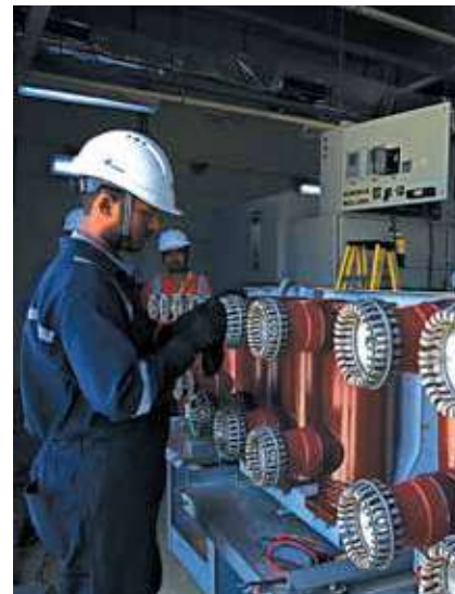
Ensuring safety standards at Cairn Oil &amp; Gas
