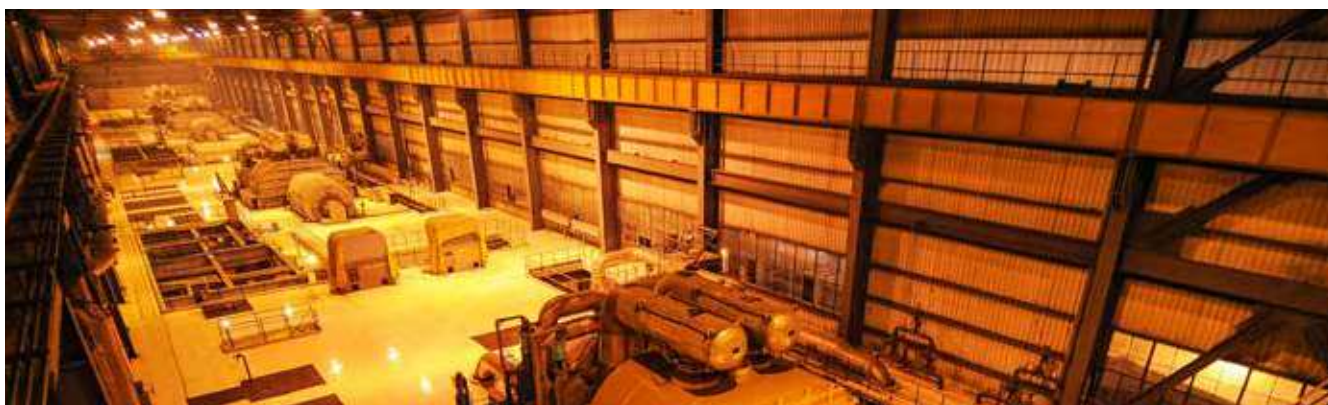
Power generation facility, BALCO
