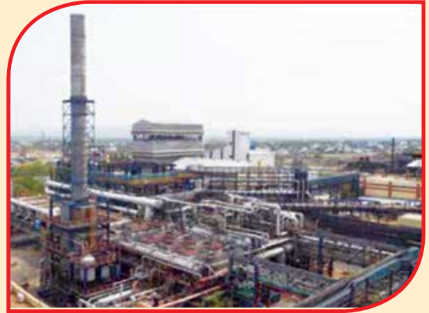
PA Plant - Ranipet, during revamp
