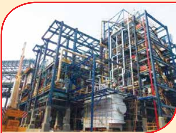
PA Plant Revamp : Oxidation Section - Ranipet
