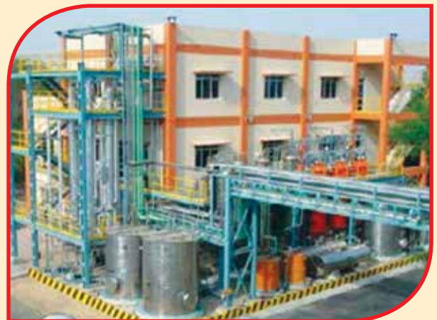
A section of the Fine Chemicals Plant
