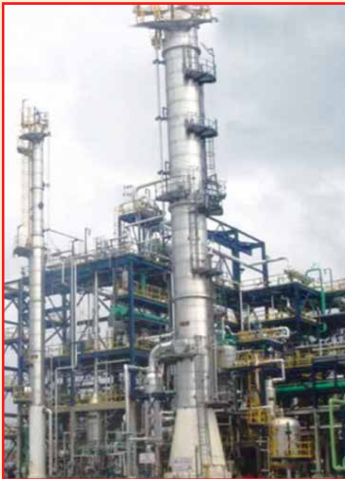
Butane Processing and Butamer Plant: Malaysia
