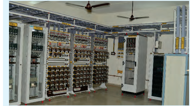
Relay Room Arrangement - Moradabad S&T Project
