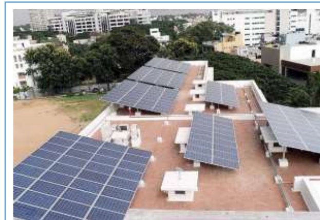
Installed Solar Panels at Surangi Unit, reducing 80 MT carbon emissions per month
