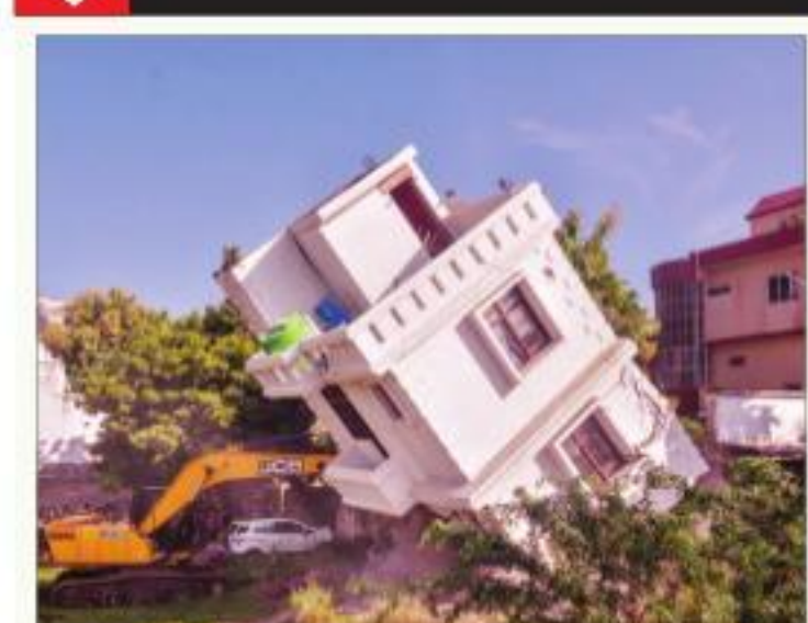
Authorities demolish an illegal building allegedly belonging to gangster-turned-politician Mukhtar Ansari, during an encroachment drive, in Lucknow, on Thursday PTI
