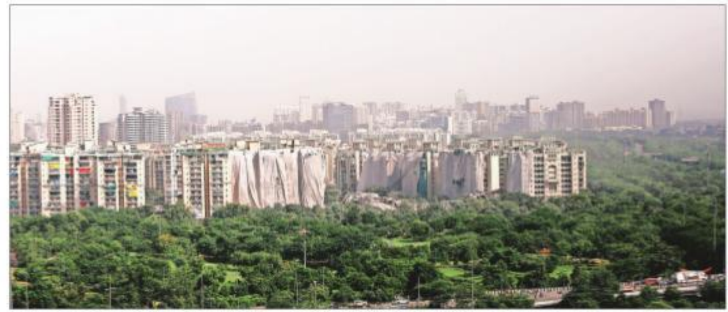
The skyline of the area in Noida's sector 93A after the demolition on Sunday. GAJENDRA YADAV
