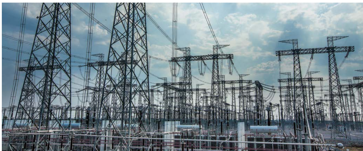
765/400kV substation commissioned by BHEL at Raichur, Karnataka
