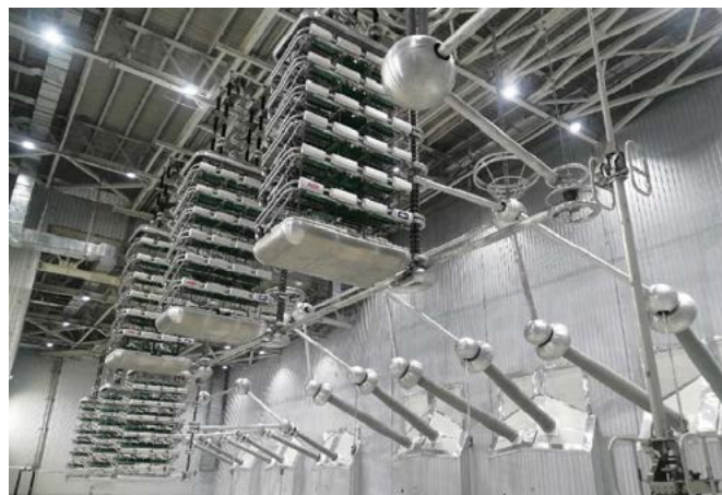
DC Hall of \pm 800 kV, 6000 MW UHVDC link between the Western Region Grid (Raigarh, Chattisgarh) and the Southern Region Grid (Pugalur, Tamil Nadu) successfully implemented by BHEL
