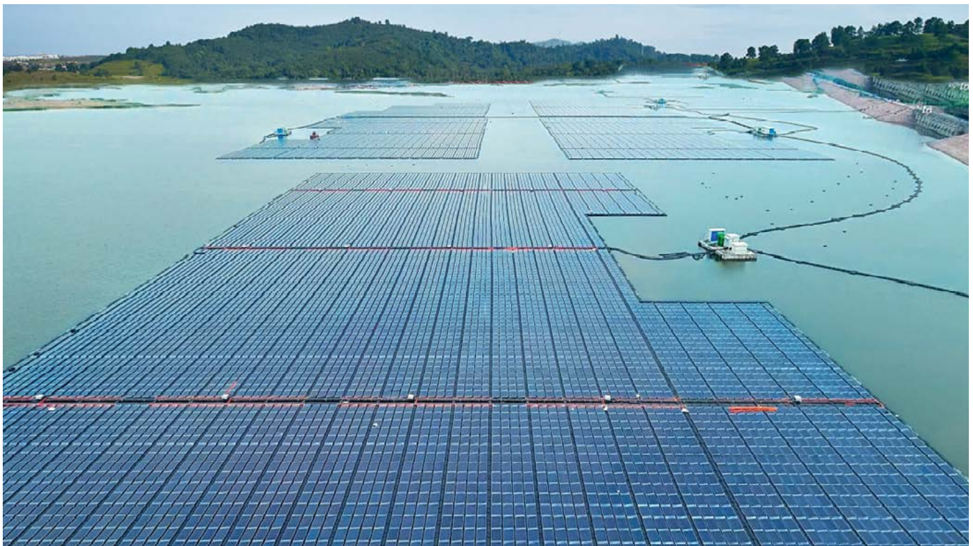
100 MW Solar PV Plant at NTPC, Ramagundam, Telangana, the largest floating solar power plant in the country, commissioned by BHEL
