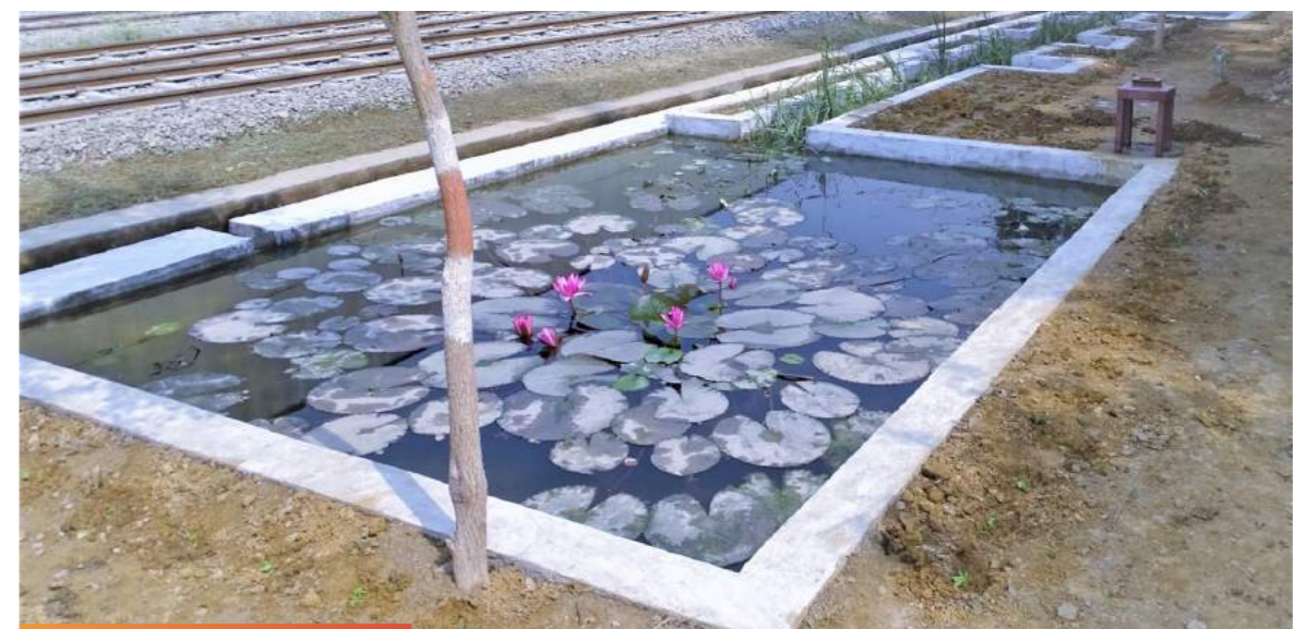
A view of the natural sewage treatment plant (STP).
