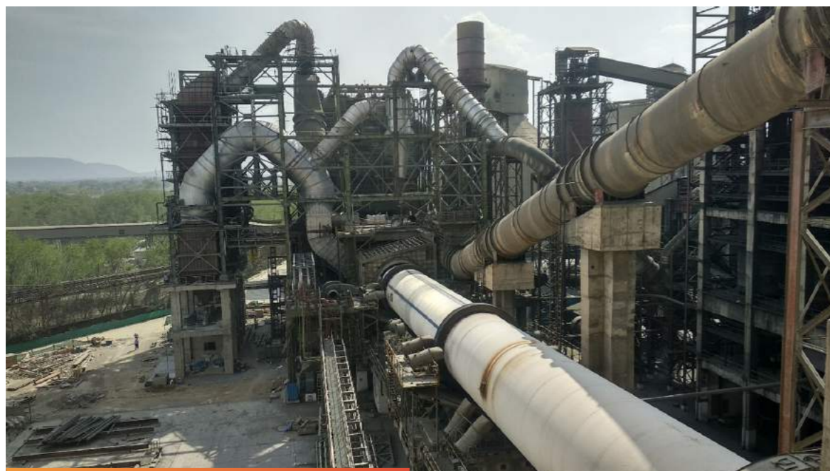
Waste Heat Recovery System (WHRS) at Satna Plant
