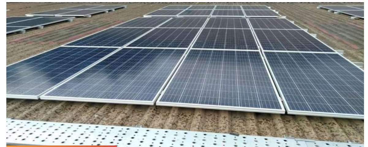
Solar Plant at H&R Johnson, Pen, Maharashtra
