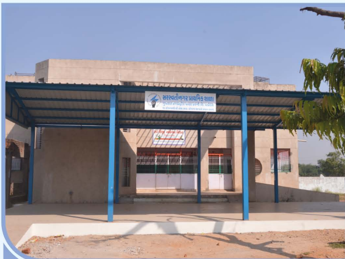
Construction of Multi purpose shed at Saraswatinagar, Primary School Village Amrol, Taluka Anand
