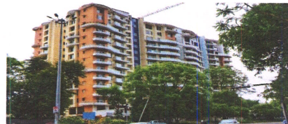
Construction of 96 flats at Tulsi Tower, Bhopal for MP Housing & Infrastructure Development Board
