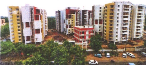
Construction of 222 Flats at Keelandev Tower, Bhopal for MP Housing & Infrastructure Development Board
