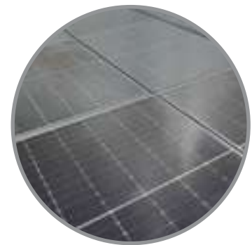
Rooftop Solar plants installed at Bajaj Allianz House
