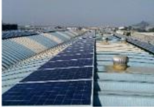
Rooftop mounted solar system
