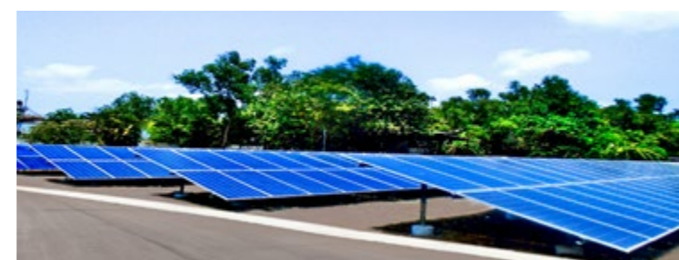
Solar Panels at Roha
