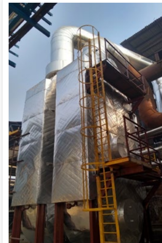
New waste heat recovery system
