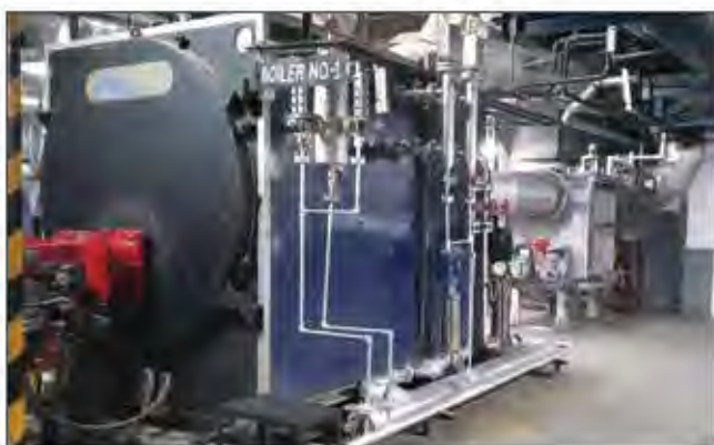
Boiler in the foreground with Economizer in the background
