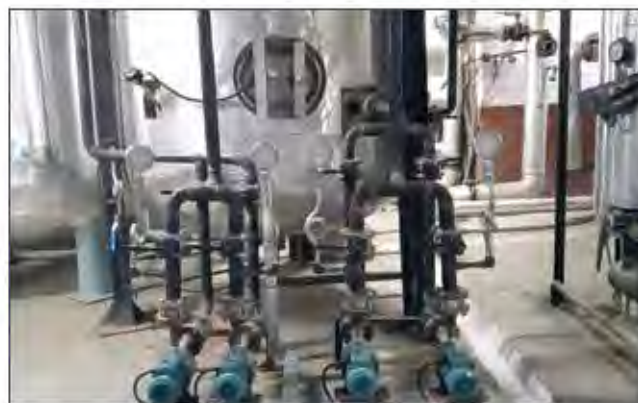
Circulation pumps with standby for hot water movement to swimming pool and rooms heat exchanger
