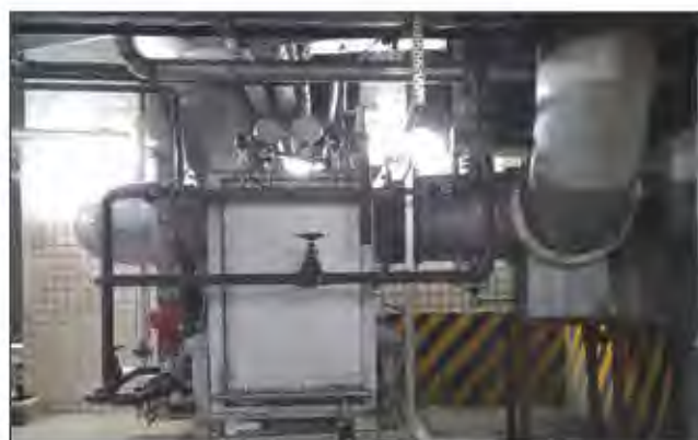
Water Pre-heater housing the ducting within its core
