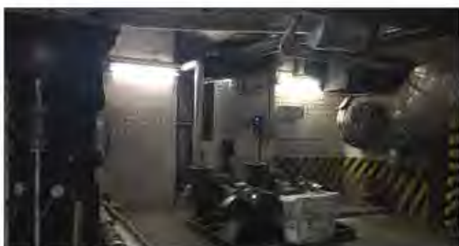
Location where the Water Pre-heater was installed
