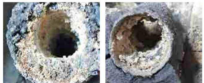
Typical Clogging Occurred
