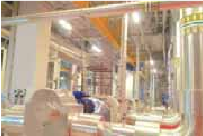
HVAC and plumbing works for Al Bayt Stadium, Energy Centre Project at Al Khor, Qatar, for the 2022 FIFA World Cup
