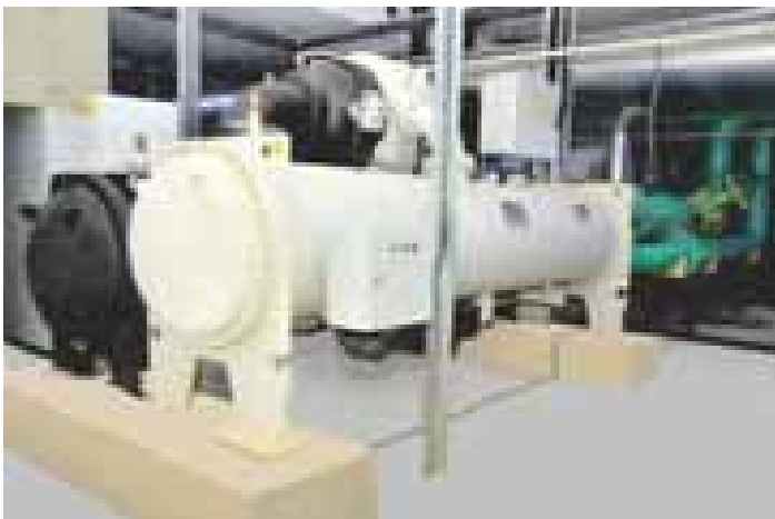
Installation of centrifugal and air cooled screw chillers, along with VRF V Plus system for Meenakshi Infrastructure, Hyderabad
