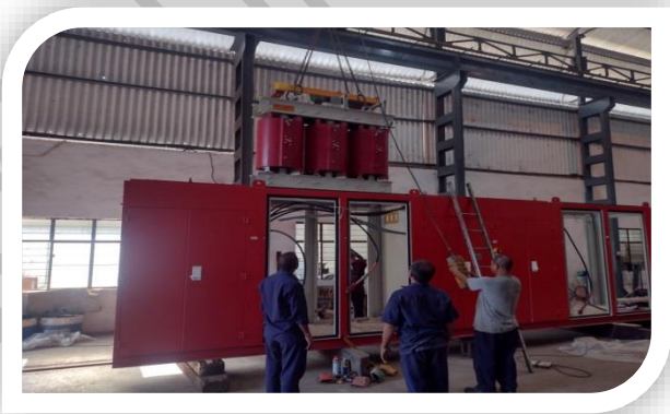
Overhaul of Dry Type Transformer
