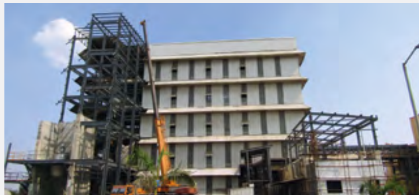
Specialty Fluorochemicals Facility (Dahej, India)
