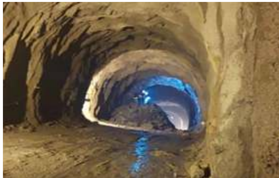
Excavation of about 11 Km in Main Tunnel of T15 completed on January 18, 2022.
