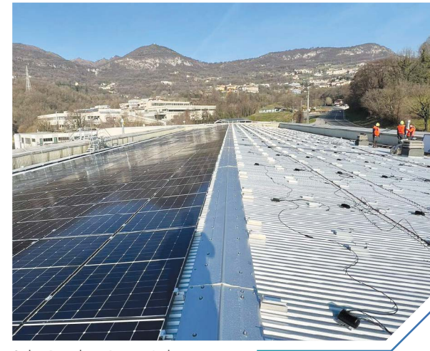
Solar Panels at Bione, Italy
