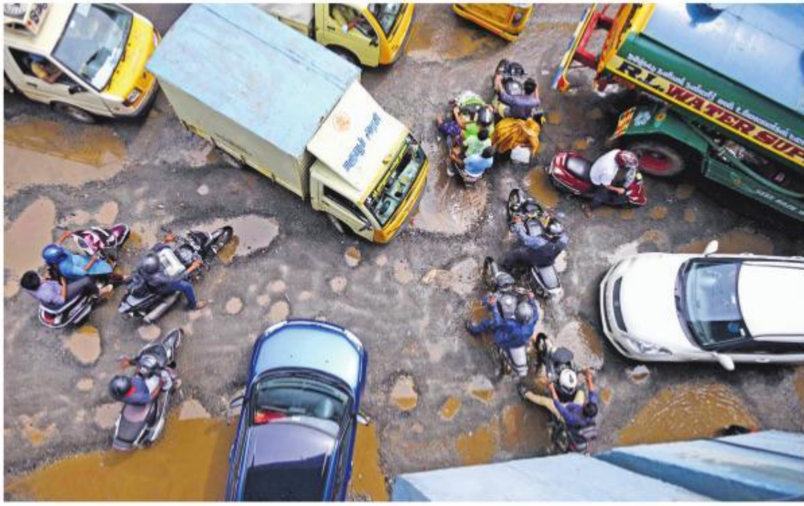
TARRED ROADS TOO MUCH TO ASK FOR? Commuters struggle to drive through a pothole-filled road at Ambattur in Chennai on Wednesday. A 32-year-old biker on Monday had hit a pothole on Anna Salai and died after being thrown under an MTC bus in the impact | DEBADATTA MALLICK
