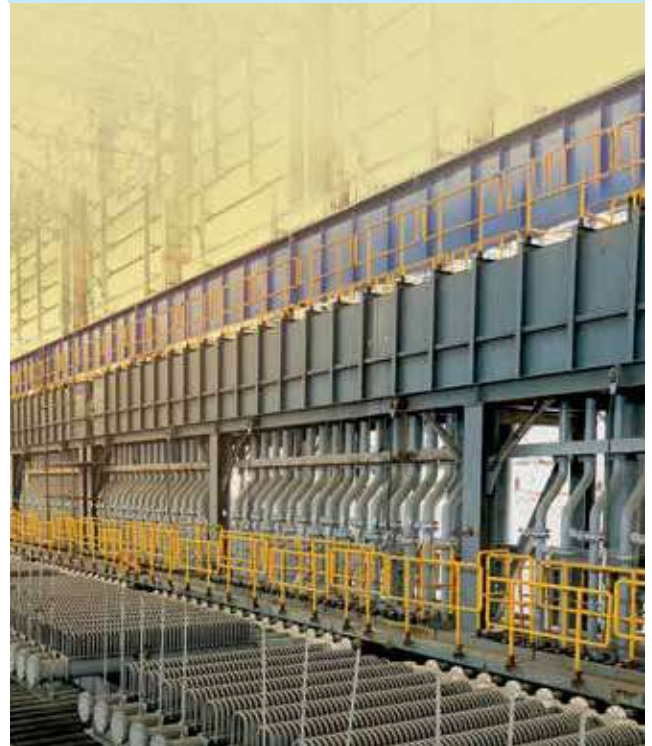
Laminar Cooling System for Rourkela Steel Plant
