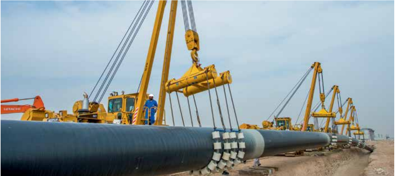
New 48" Crude Transit Line from North Kuwait to CMM (TL-5) Project for KOC, Kuwait
