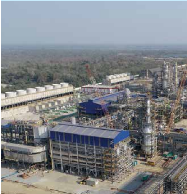
Ammonia-Urea Plant for HURL at Sindri, India
