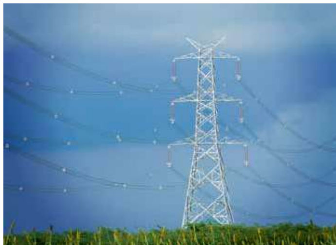
400kV Kamudhi-Ottapidaram Transmission Line, Tamil Nadu
