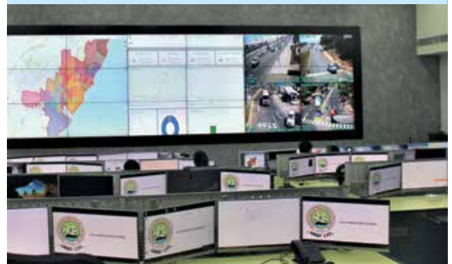
GVMC City Operations Center
