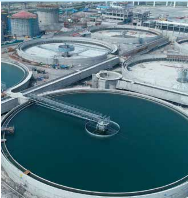
318 MLD Coronation Pillar Sewage Treatment Plant, Delhi
