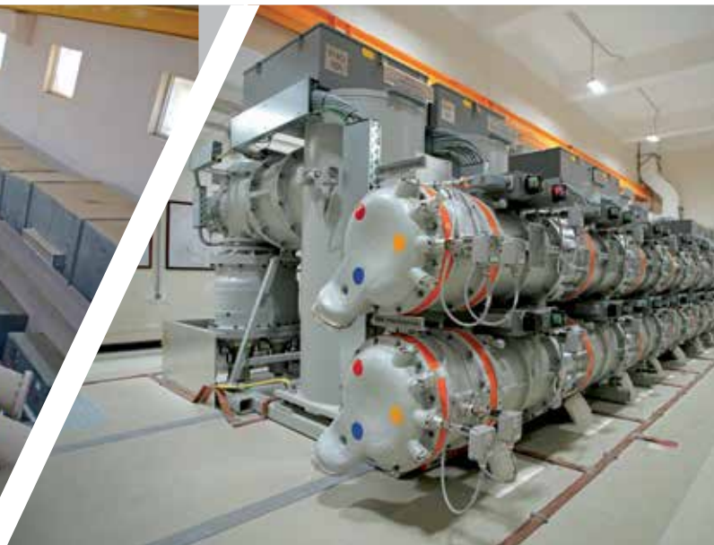
132-11 kV Umm Beshar and 132-11 kV Wakrah-4 Substation
