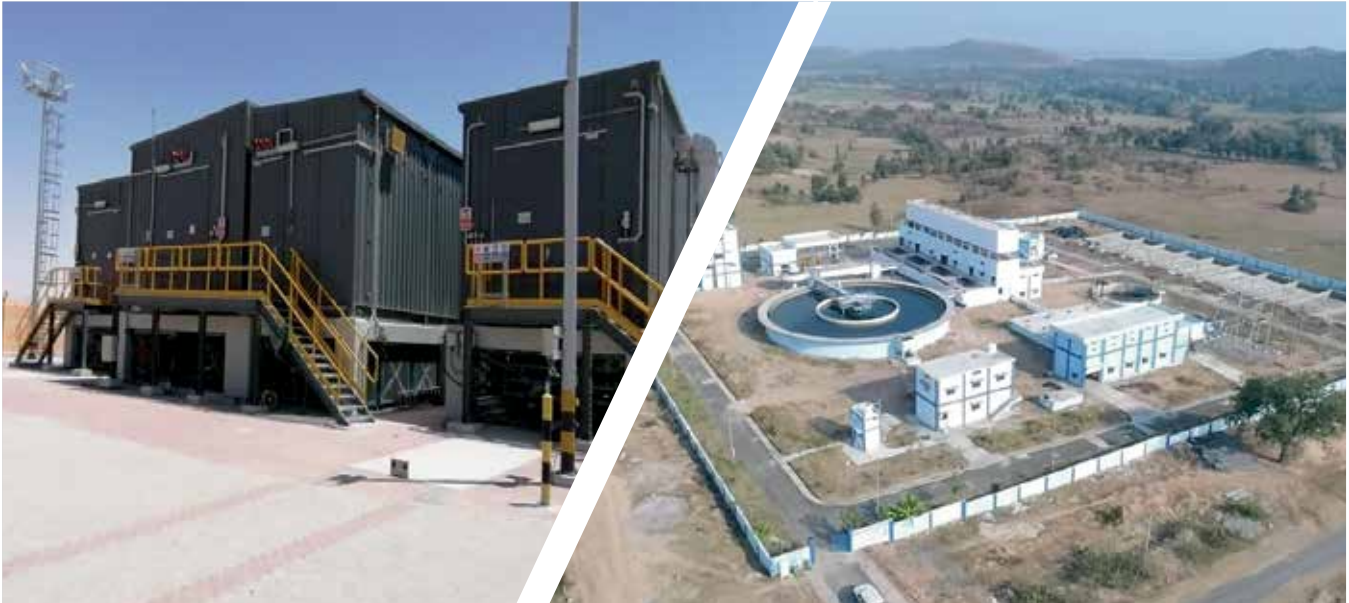
Haliba, Containerised Substation
