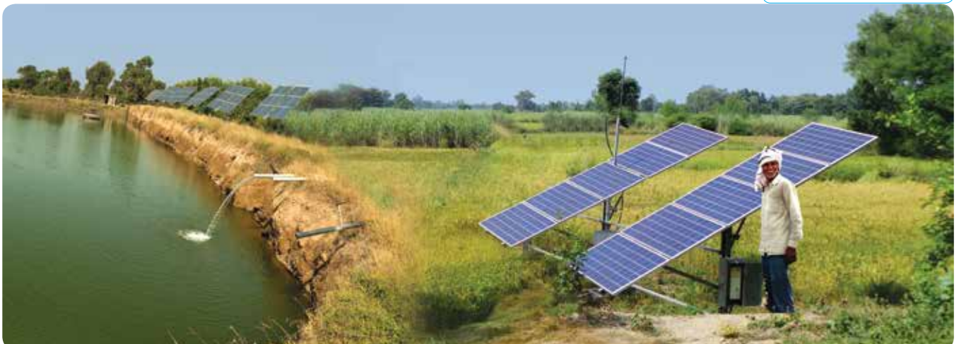
Solar powered drip irrigation in agriculture farm.
