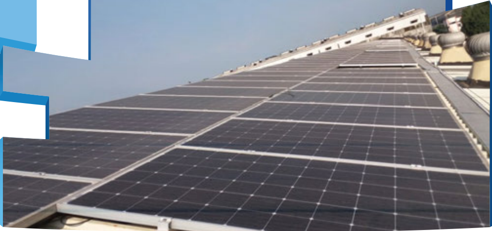
Solar panels installed at the Dadra plant ▼
