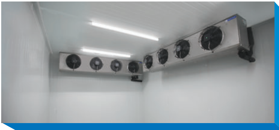
Inside view of the cold room supplied and installed at the Municipal Corporation of Greater Mumbai (MCGM), to store vaccines as a part of Vaccine inoculation program
