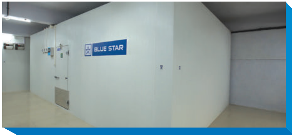
Meher Distributors Kalher, Thane, where Blue Star supplied and installed cold rooms for Vaccine Storage
